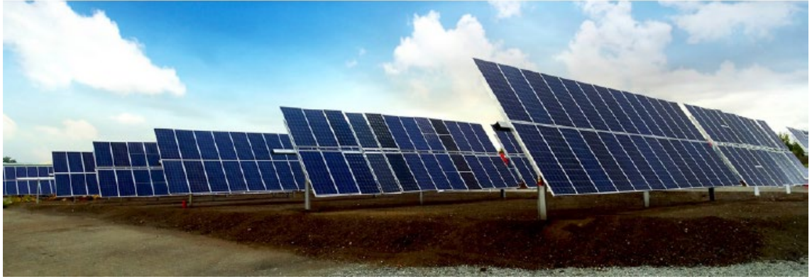
Figure 4.1: Typical Tracking Panels
