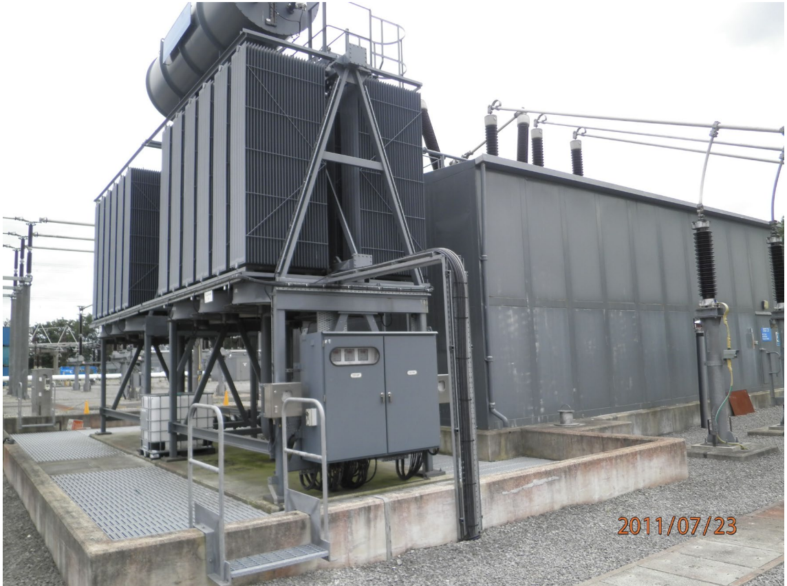
Figure 4.3: Typical (large 400kV) Power Transformer
